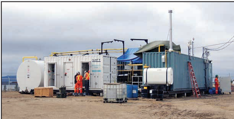
Colville Lake new hybrid power plant.
